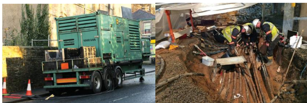
Figure 3-24: Response required due to substation flooding 23
